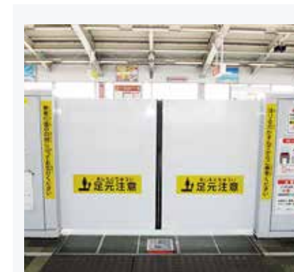
Platform doors (movable safety barriers)
